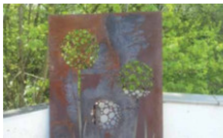
Black discolouration caused by air pockets and moisture on the fresh surface.
