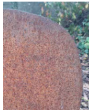
An example of a weathered surface after more than three years.
